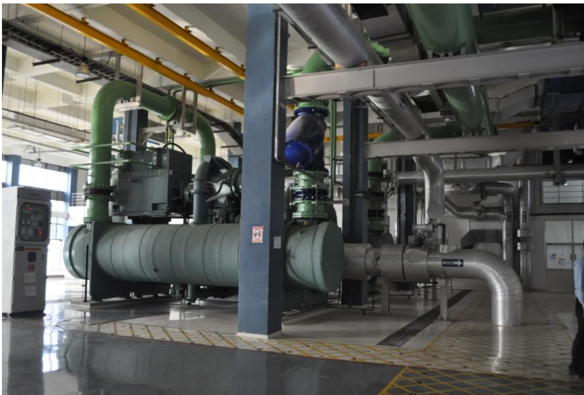
District cooling system
